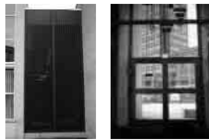
Exterior and interior views of the perforated metal that hides the glass emergency exit at the Academy in Rotterdam.
